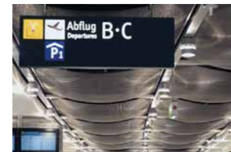
Ceiling elements with sag. Terminal B, Düsseldorf Airport, Germany.
